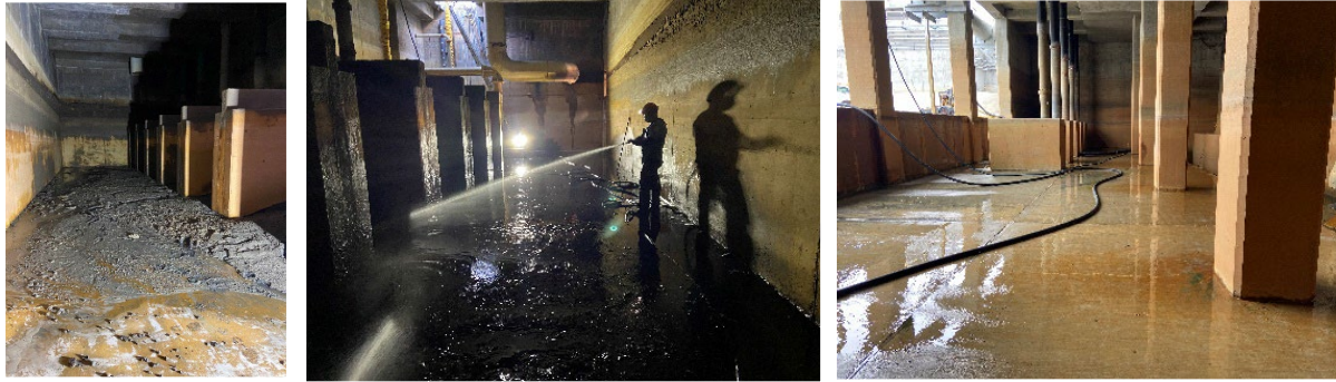
Photos (Left to Right): Holding Basin No. 4 wet well before cleaning, during cleaning, and after cleaning.
